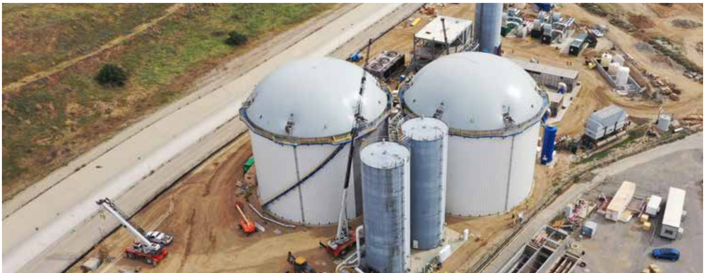
Anaergia’s high solids digesters at the Rialto Bioenergy Facility process three times higher throughput than conventional digesters.
