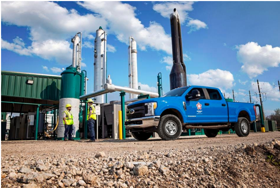
RNG-to-energy plant at a Republic Services Landfill Site. REPUBLIC SERVICES
