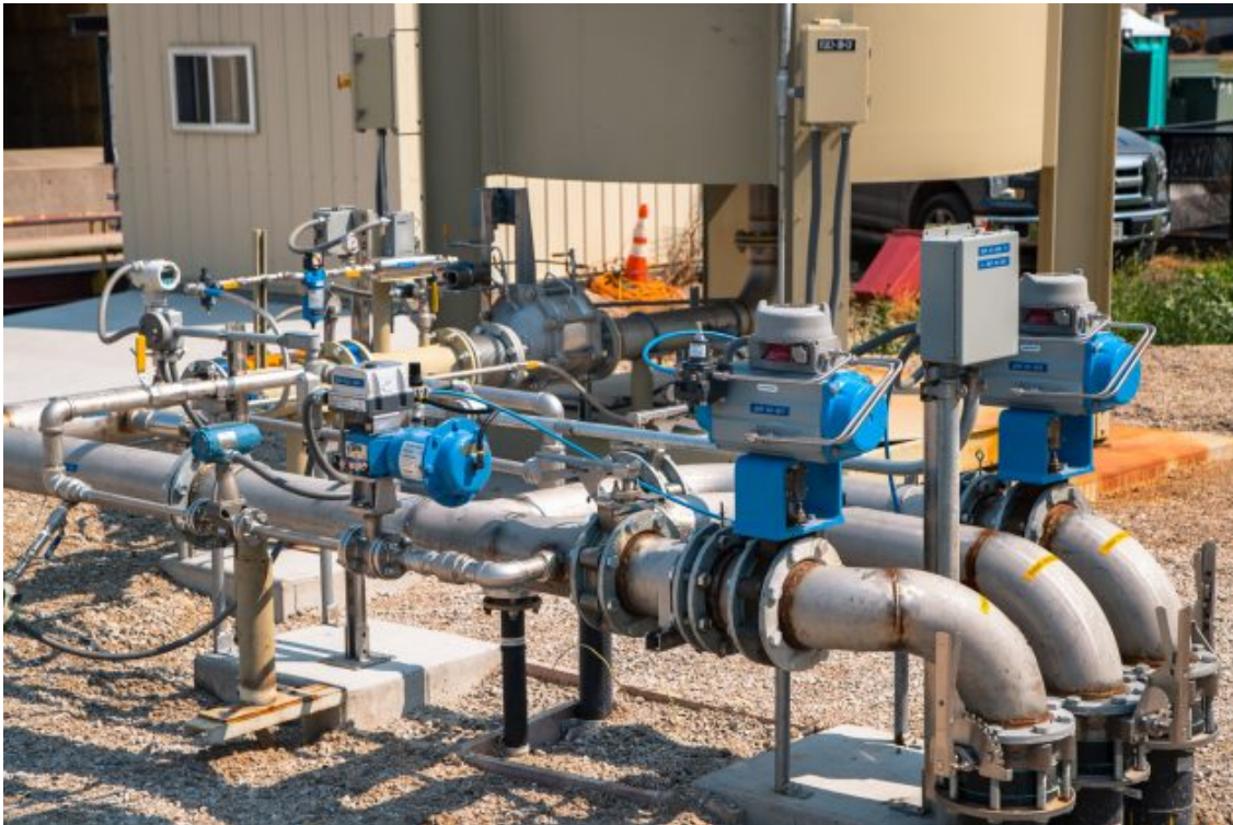
Biogas is injected into the natural gas pipeline network as renewable natural gas (RNG). (Image Courtesy Of US Grain)
